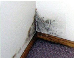
Condensation has led to mould problems on the drywall.
