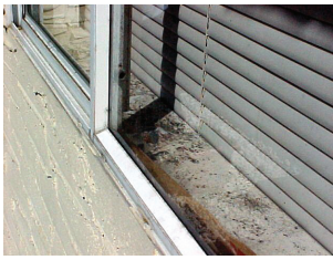
Evidence of problems resulting from condensation can be seen on the interior window sill.
